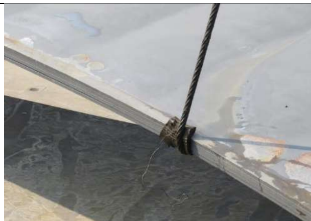
It is recommended to use suitable edge protection when wire slings are used for handling the cargo.
