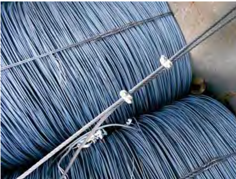
✘ Incorrect use of bulldog grips
