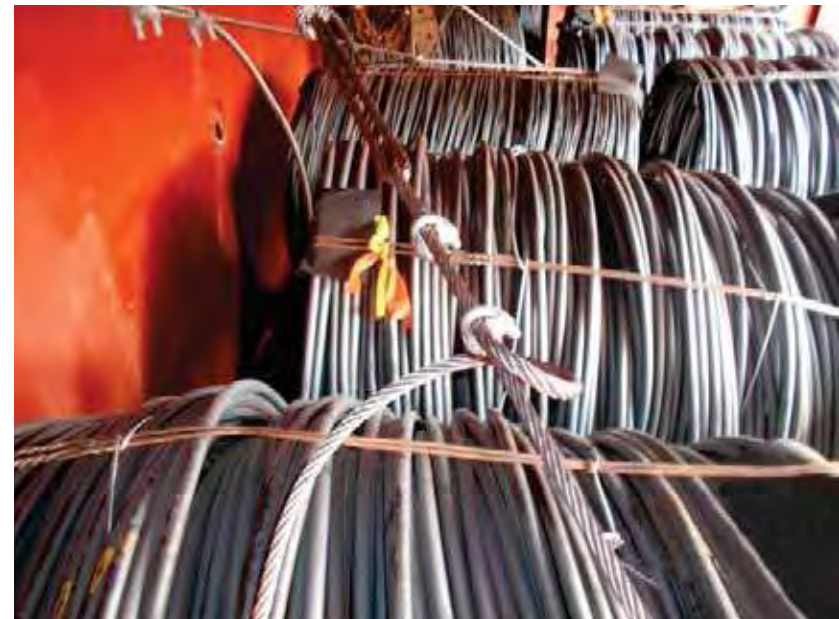
✘ Incorrect use of bulldog grips with grips on the live wire. Insufficient number of grips used
